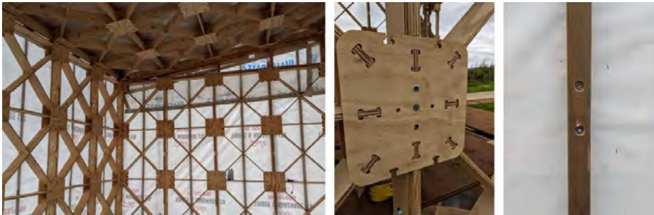
Figure 3. Synthetic Building Wrap (non-woven thermally bonded polypropylene) over the modular frame (left), the cavity batten mounting points (middle) and the batten installed (right).
