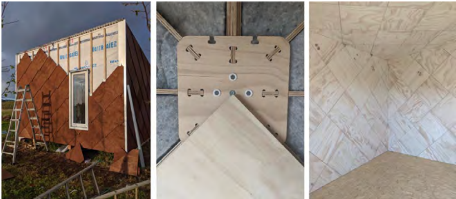
Figure 4. Installation of the Thermally Modified Plywood Cladding (left), a close up image of the pressure clip receptacle used for the internal linings (centre) and the finished lined interior (right).
