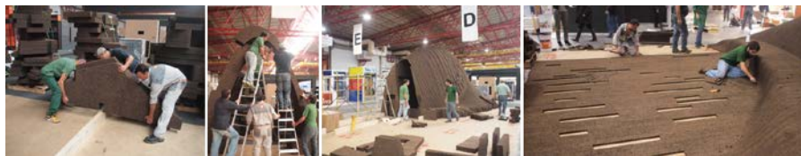
Figure 4. Placement of arch base in wood billet; arch keystone placement; vault construction; flooring with gaps for turf rolls (photos by PAV)
